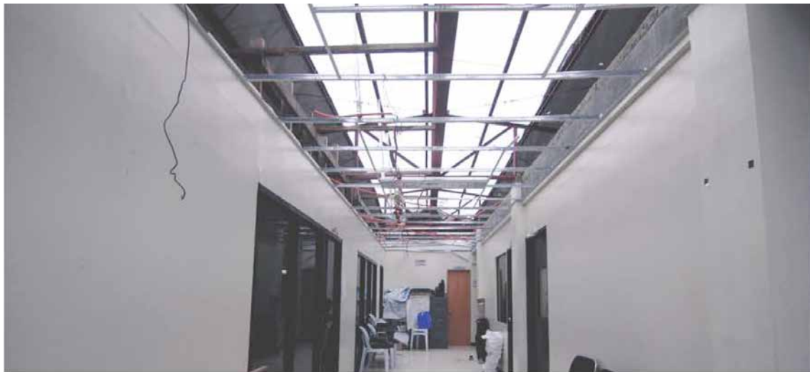
Fig. 46: Roof damage at Tacloban main health center (World Health Organization)
