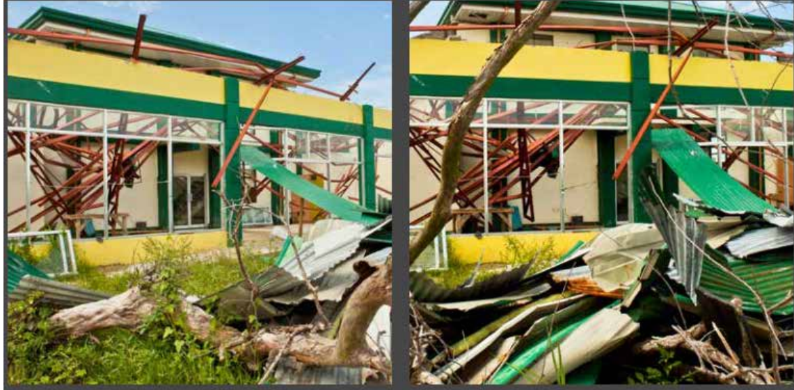
Fig. 45: Collapsed structures of Leyte Provincial Hospital (World Health Organization)
