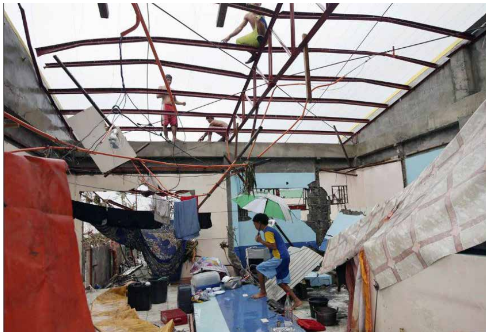
Fig. 42: Collapsed roof (NBC News, 2013)
