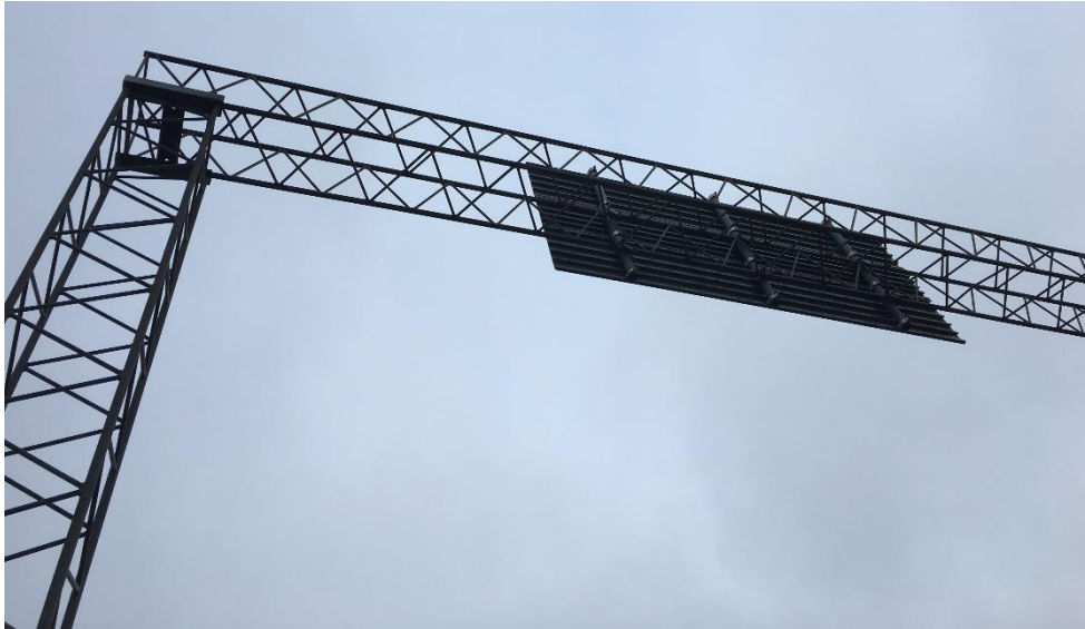
Figure 3.3 A Swedish highway truss portal carrying a road sign. This one found near the Axis Headquarters.
