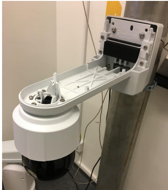
Figure 3.17 An PTZ camera fastened on the bottom part of the Connect arm that is mounted to the Big Hug pole mount.
