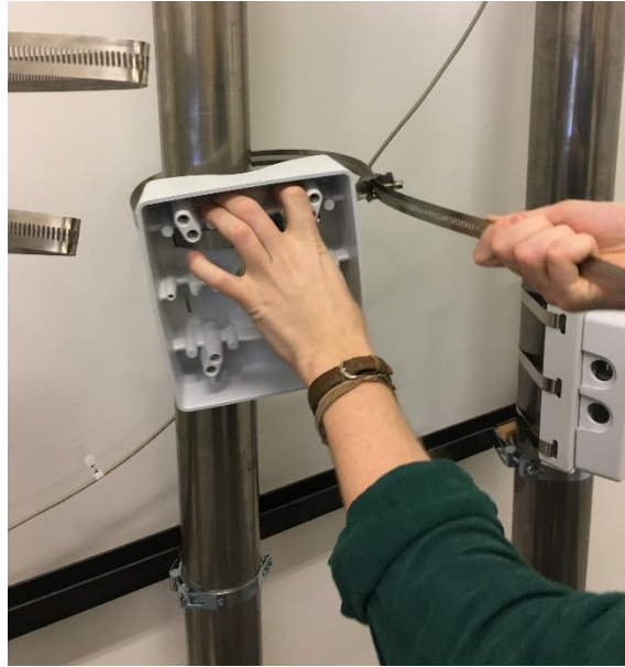
Figure 3.16 During the installation test of Big Hug many frustrations were expressed with the metal straps.
