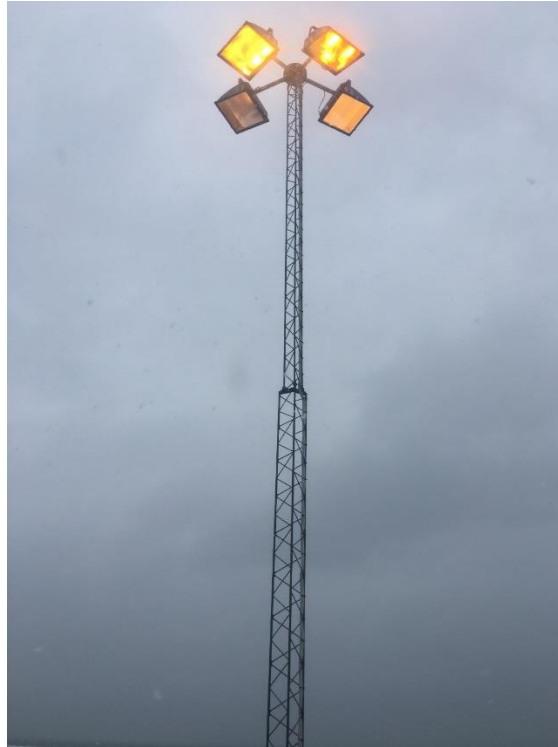
Figure 3.2 A typical harbour truss carrying lights, this one found in the Port of Trelleborg.
