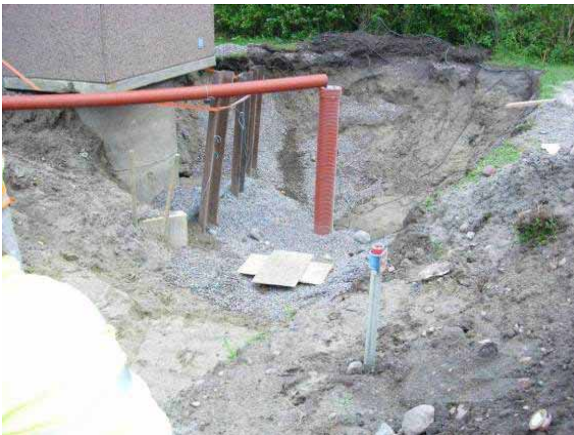
Figur 4.11 Västra Gryet – pumpstation, pumpning
