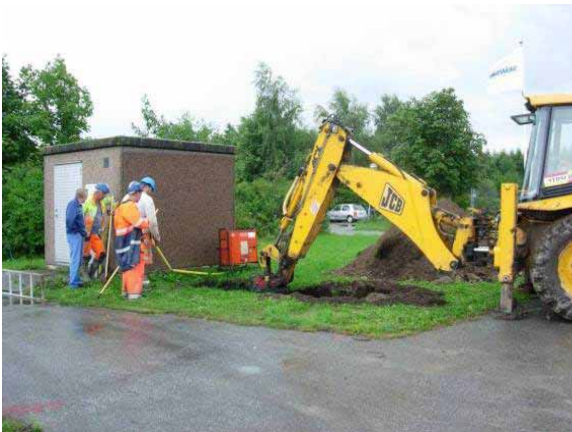
Figur 4.7 Västra Gryet – pumpstation
