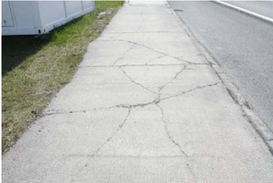
Figure 3-19 Worn pavement at Grensásvegur
