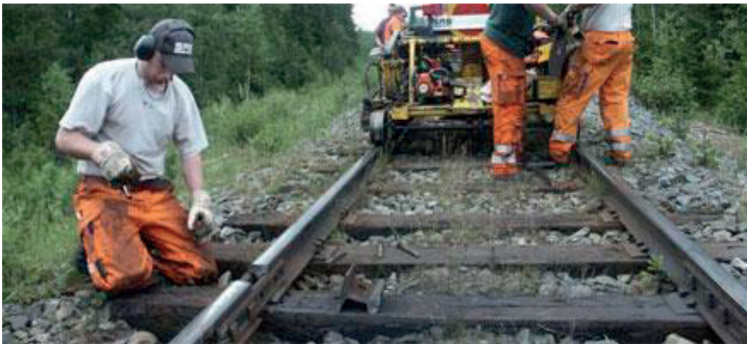
Figur 30: Rälsbrott (Trafikverket, 2012d).
