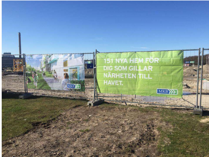
Figure 5-2 On-site promotional material at Sluringen mentions "151 new homes for those who like proximity to the sea"
