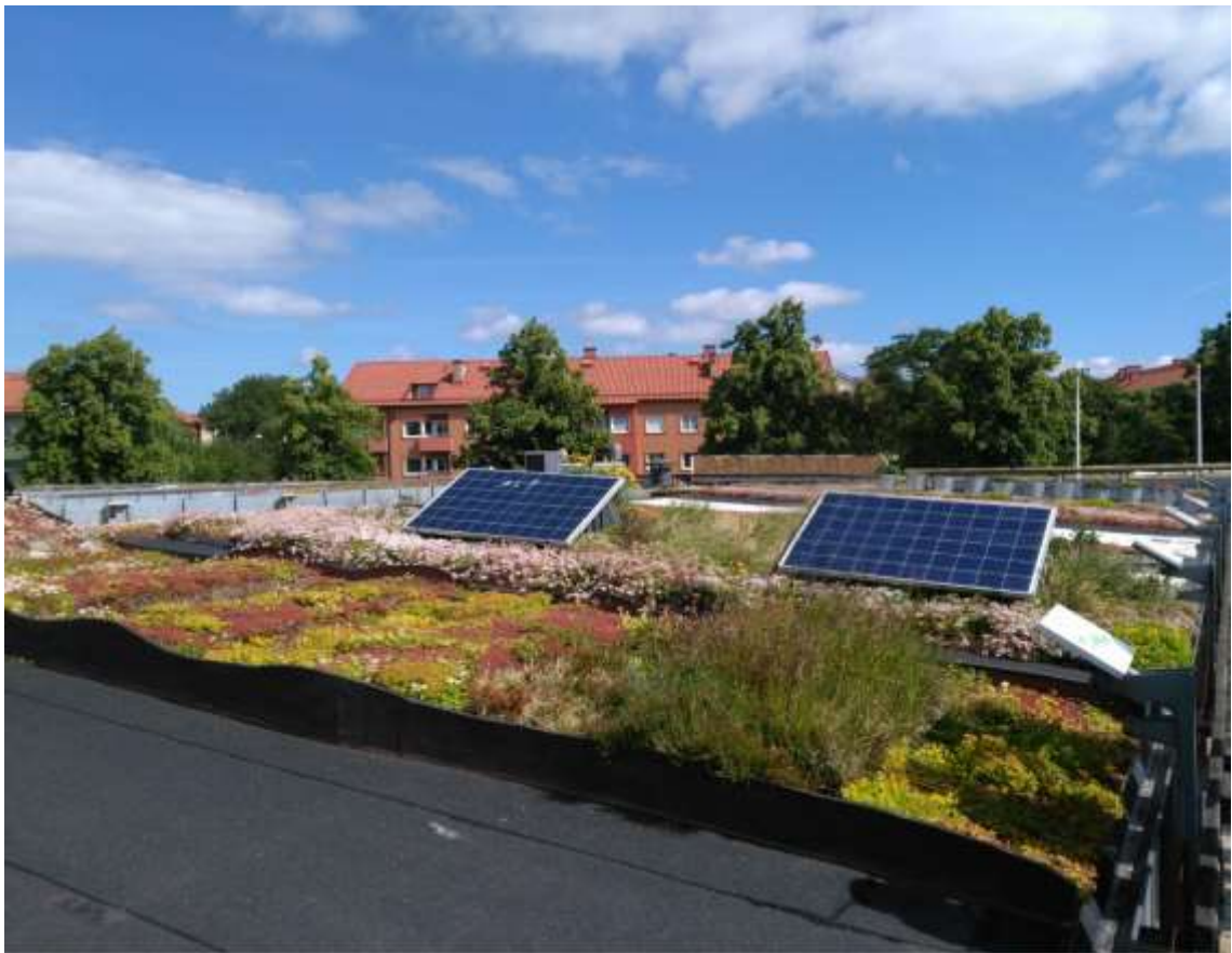
Figure 4-8: Green roof with solar panels in Malmö
