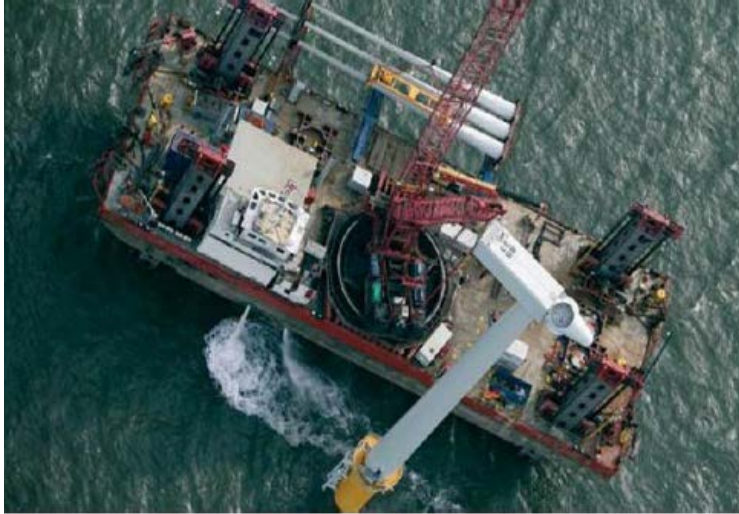
Figure 12. The jack-up barge Sea Jack is in the higher end of sizes (Assessment of vessel requirements for the U.S. offshore wind sector, 2013)
