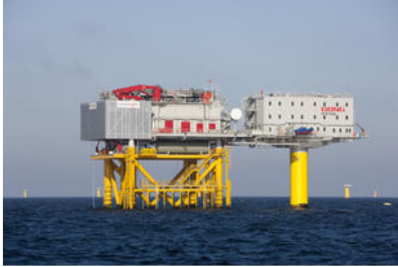
Figure 7. The transformer station and permanent accommodation at Horns Rev 2. (Oglaend System, u.d.)
