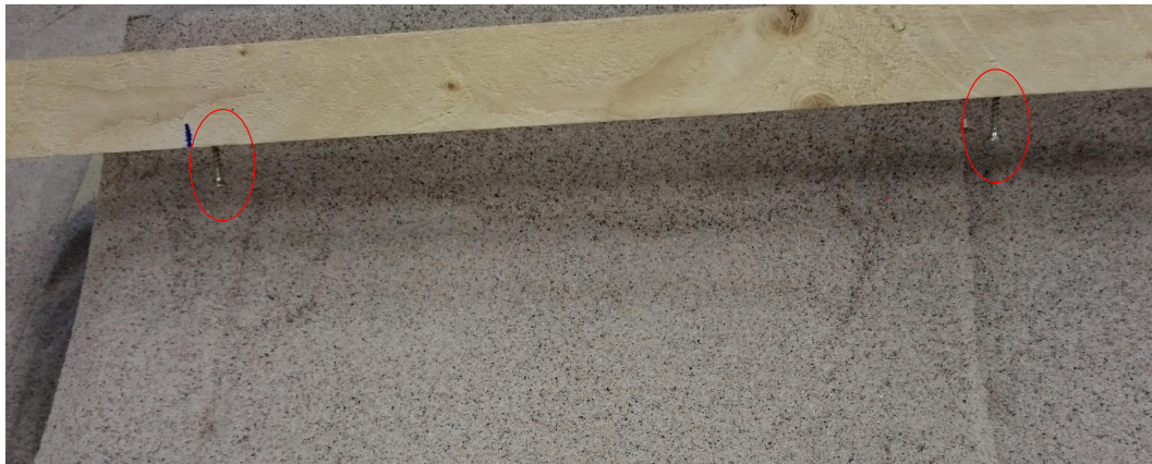
Figure 4.6: Guiding board with two 2 cm long strews that helped distribute the sand layer evenly over the entire roof
