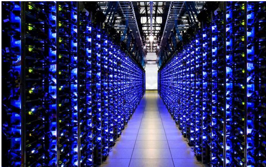
Figure 1: Photo from inside a data center. Source: [ http://www.bloter.net/archives/150382 ].
