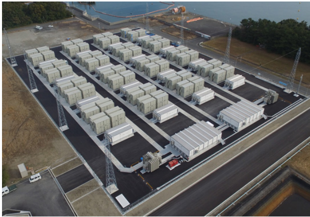
Figure 27: Buzen substation in Japan, 50 MW & 300 MWh
