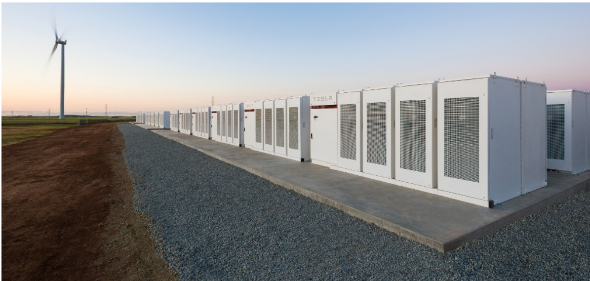
Figure 26: The Hornsdale Power Reserve in Australia
