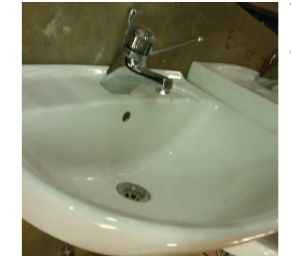
WASH BASIN & TAP FOR BATHROOM
