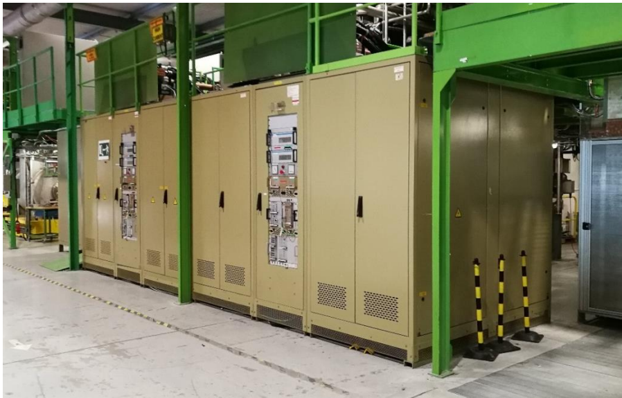
Figure 3 - 2x10 electrical cabinets – picture from one of CERN facilities
