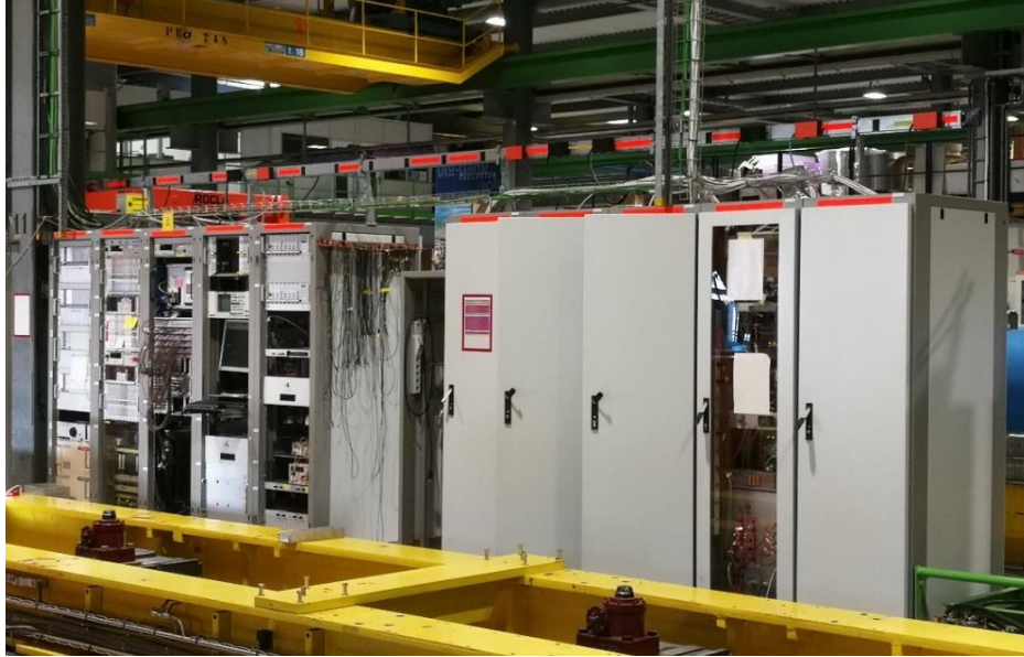
Figure 2 - Open/closed cabinets + racks in a row – picture from one of CERN facilities
