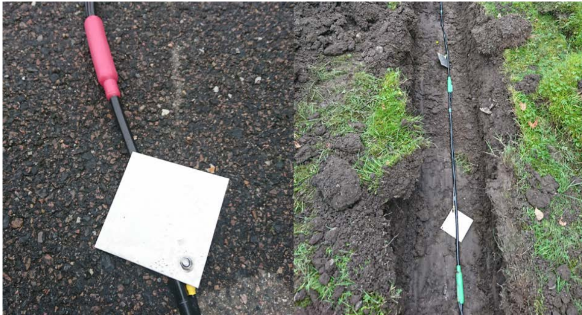
Figure 27. The left image displays the stainless-steel plate-electrode used at the Alingsås site. The right image indicates the electrodes were installed in the excavated trench at a depth of 40 cm.
