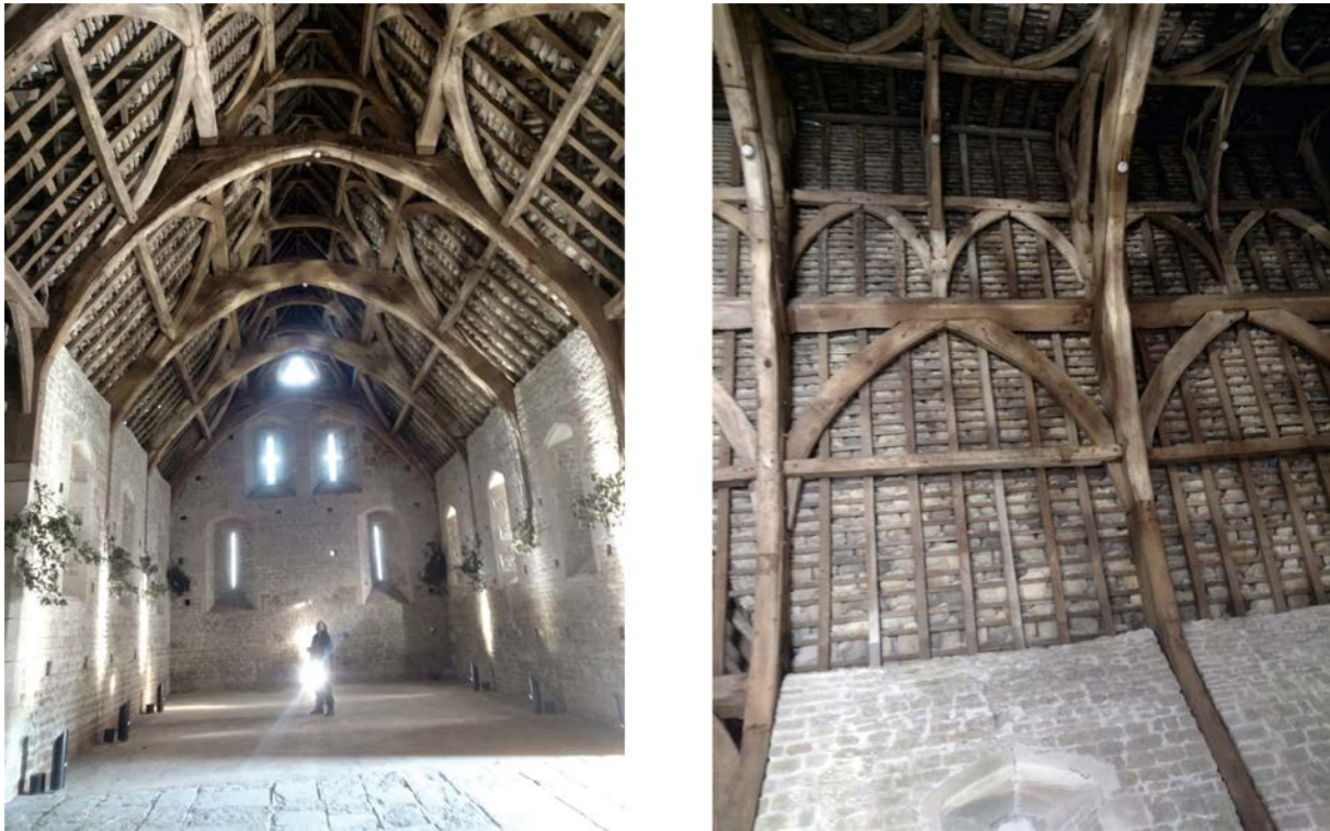
Figure 31. The original 14 th century timber frame roof structure of the Glastonbury Abbey barn. (Photo: author)
