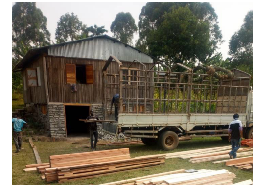
24. The bungalow is dismantled before the transportation to the island to be reerected.
