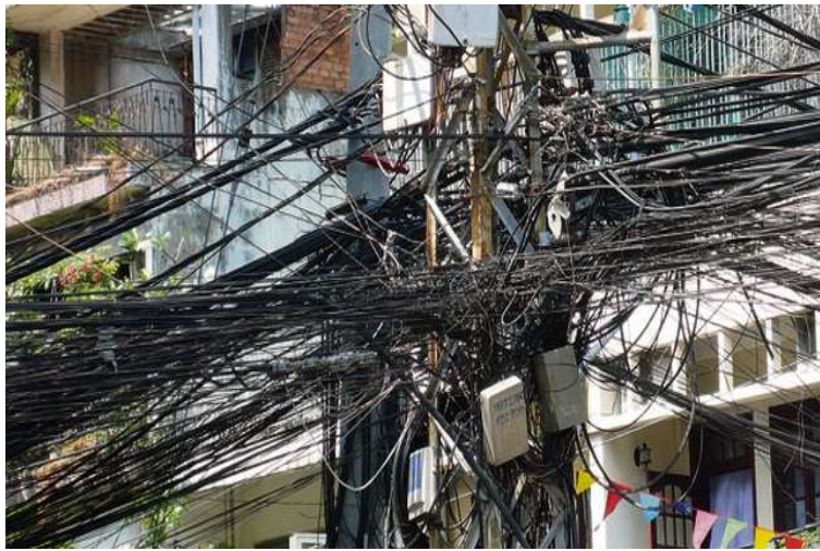
Figure 81 - Typical electrical post wiring nest in informal settlement areas. Illegal connections (aka "jumpers") are a common occurrence and source of ignition in Quezon City.
