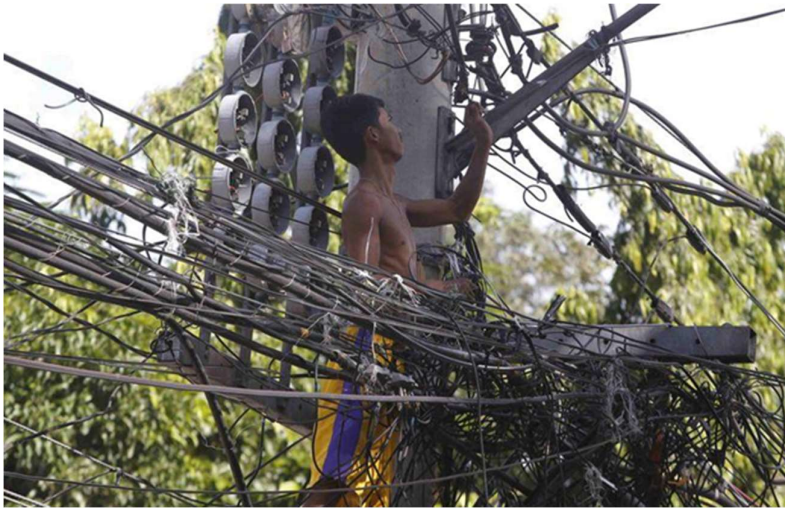
Figure 33 - Illegal electrical connections ("jumpers") is a common issue in Quezon City. (credit: REUTERS/Erik De Castro)
