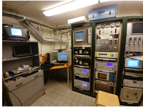
Figure 29: Underneath the tower is the control room which houses all the instruments.
