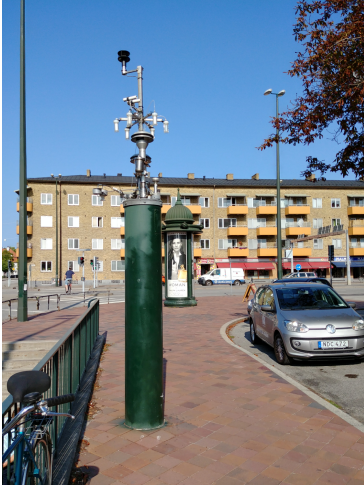
Figure 28: The measurement tower that protrudes from the ground has all the measurements station's sensor inlets for the instruments. The cables are routed directly below the ground.
