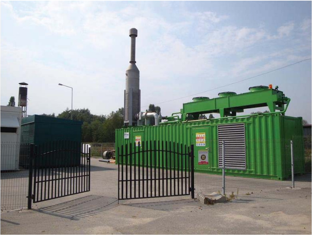
Figure 7. Combined heat and power plant from landfill gas (SPSEP).
