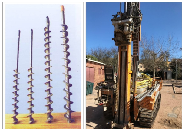
Figure 4.1. The screw augers of the different sizes, (left, SGF, 2013); a drill rig with the lifted screw auger (right). Photo by the author (2018)
