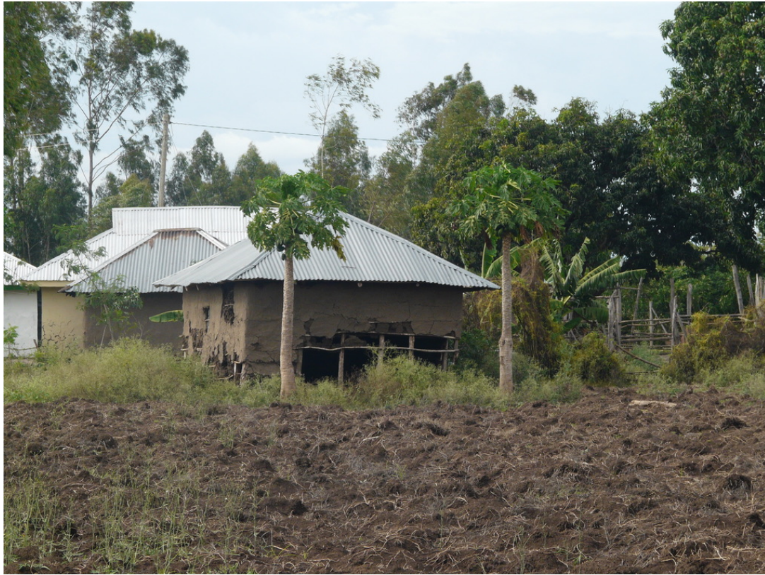
Figure 13. House damaged by floods.
