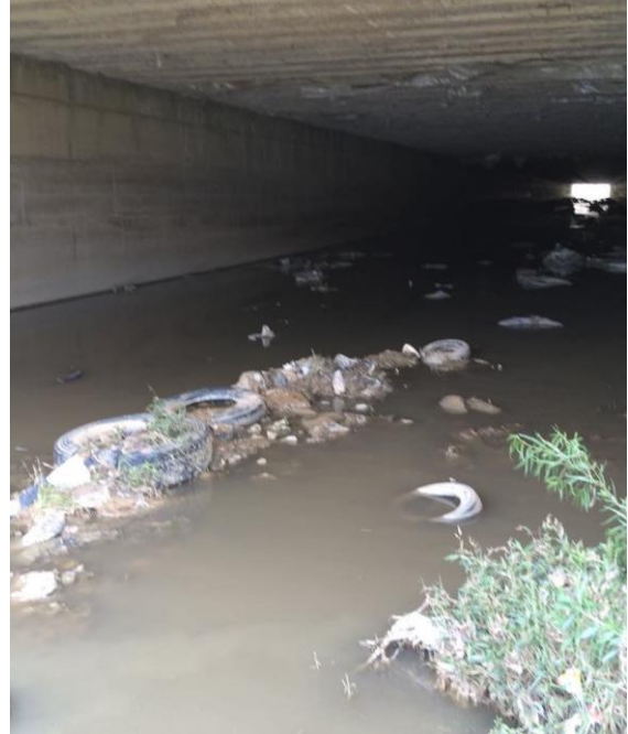
Figure 5.6 Solid waste in Rocha River under Puente Cajón (ID 3).
