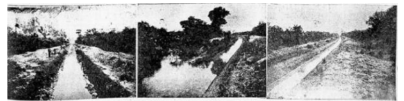
Project for straightening the Belém river, from 1933. Picture from Jornal Correio do Paraná
