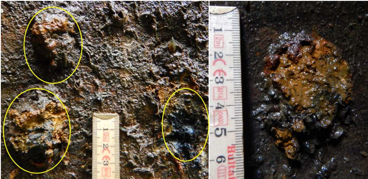
Fig. 6.1. Rust nodules covered with mainly red rust at a concrete wall in the field locality of The Sound. Generally these had a diameter of three to five centimeters. These are slightly covered by the surrounding biofilm.
