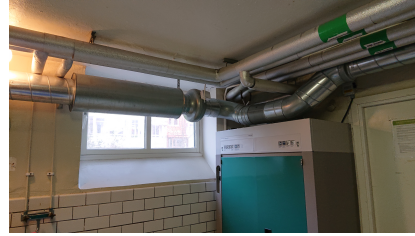
(b) The noisy pipes in the laundry room
