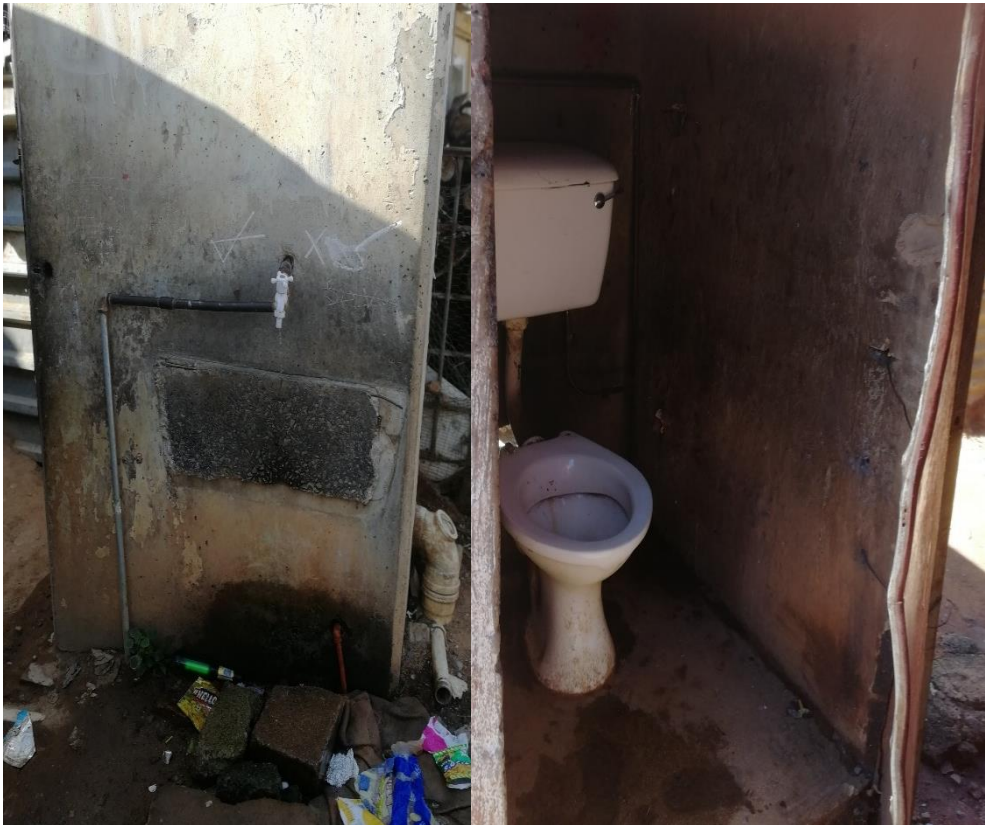
Figure 14: Cistern-flush toilet at Zandspruit.
