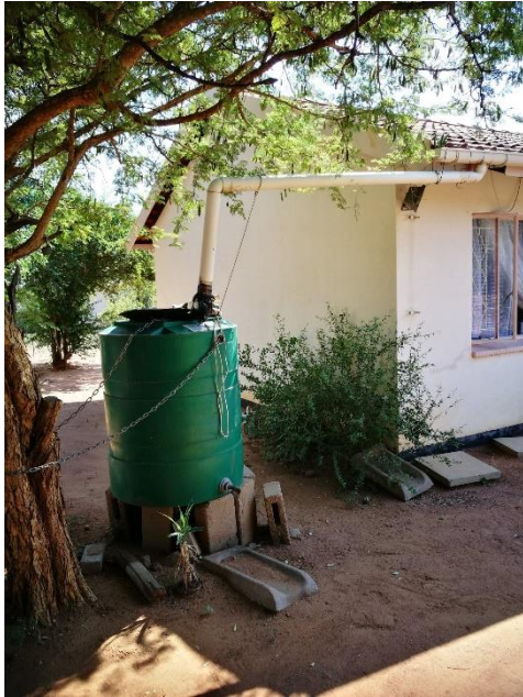
Figure 11 (L): JoJo Tank for Rainwater Harvesting
