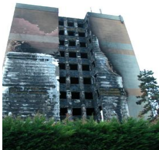
Figure 7 Façade fire in Dijon, 2010 [21]
