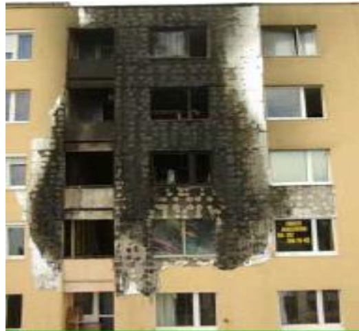
Figure 6 Façade fire in Miskolc, 2009 [19]
