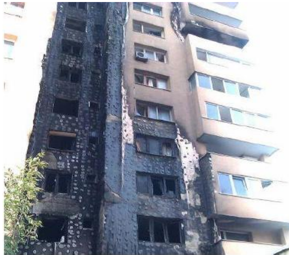
Figure 8 Façade fire in Târgu-Mureş, 2012 [22]
