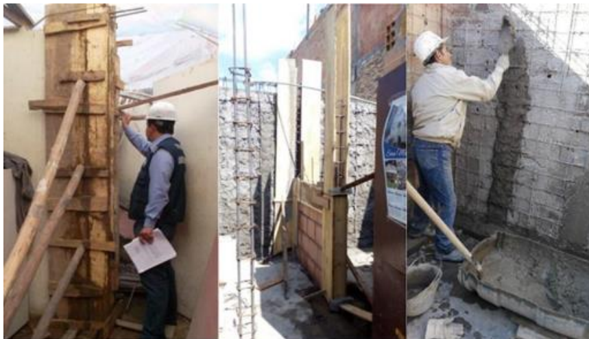
Figure 16: Casting of column, masonry of additional inner wall, metal mesh with plaster. (Build Change, 2018)
