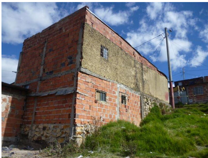
Figure 13: Inadequate confined masonry with poor connections (Acevedo et al. 2016)
