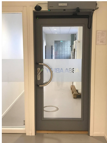
Figure 2.13: The old safety sensor is the long black sensor attached to the top of the door leaf. The grey box mounted on the wall is the operator. The little black sensor attached to the left of the operator is the activation sensor.
