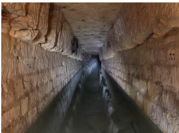
Figure 9: A flooded gallery (Credits: Zul, https://www.zul-photo.fr/zul-photo-accueil/sous-les-rues-catacombes/ )
