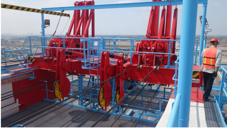
Figure 8: Shows how the hydraulics is mounted on the STS-crane.
