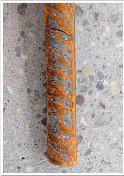
(a) Crack at gripping area. Machine jaw marking just over ribbing area.
