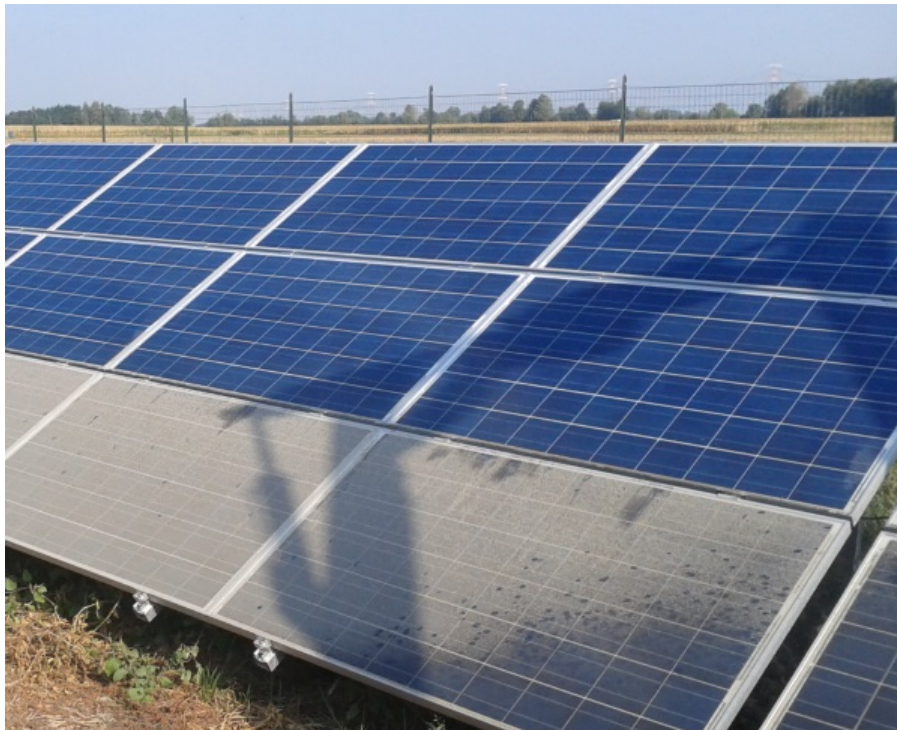
Figure 1.4: A visualization showing clean panels (top) and soiled panels (bottom). (Source of image: http://pannelplus.divegroup.it/zh/press_scheda.aspx?press=9 )
