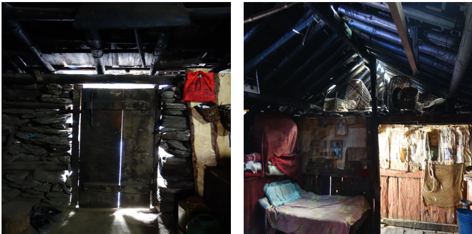
(a) Gaps around a door.
