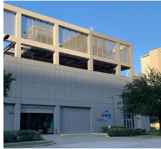
Figure 4-8: Houston Union Station District Cooling Plant
