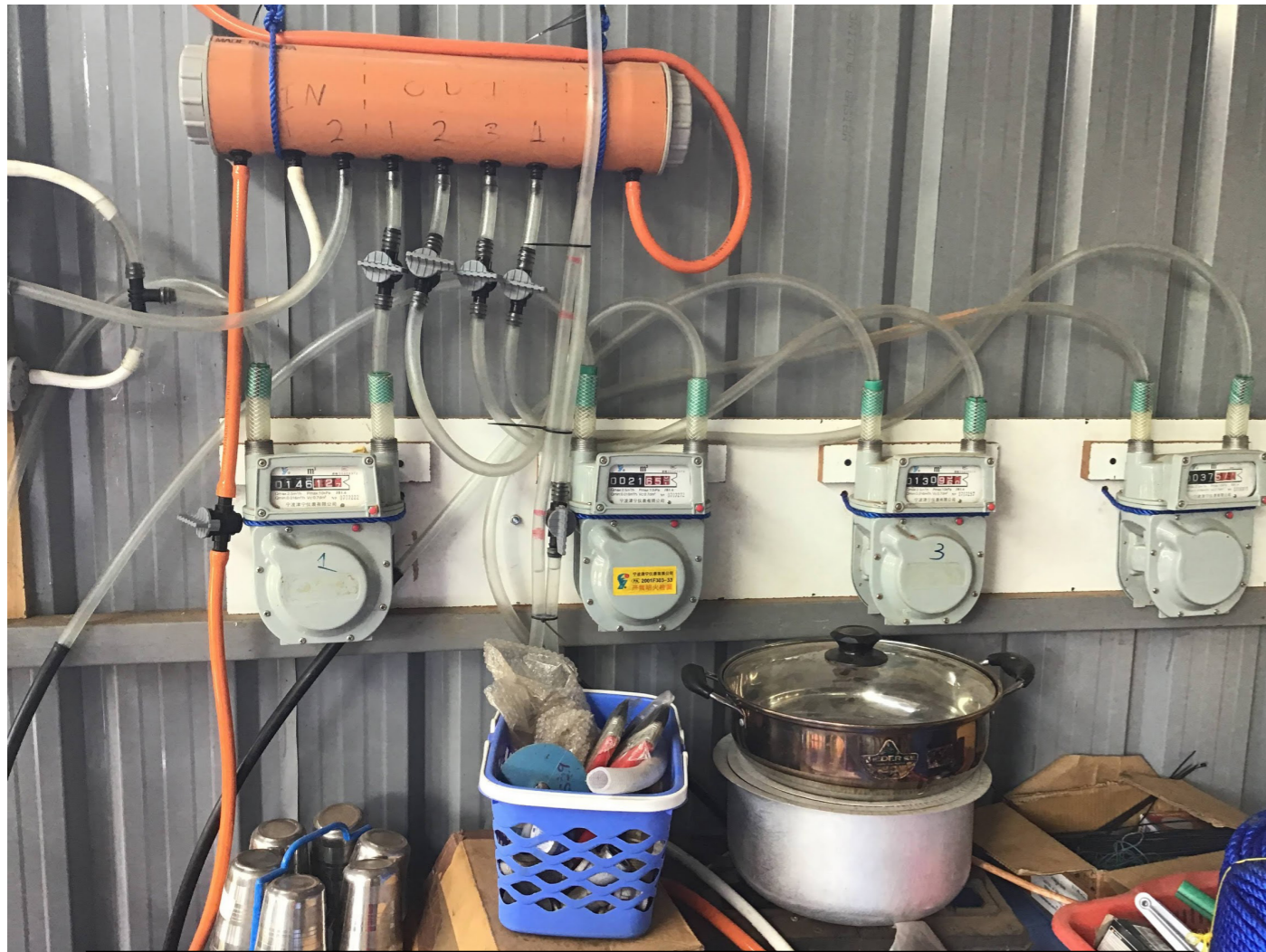
SOME OF THE HARDWARE AND TESTING SETUP BEHIND THE DUNGA BEACH BIOGAS SYSTEM.
