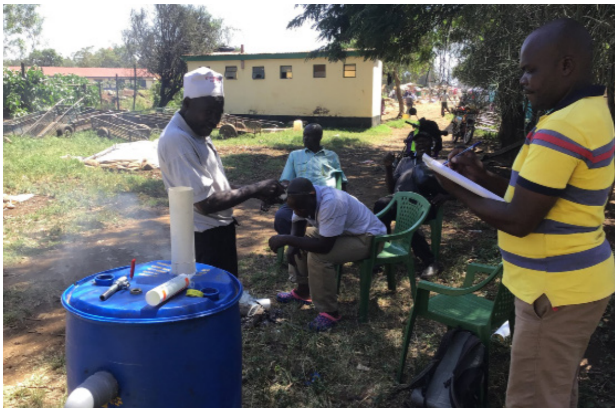
MEMBERS OF KIBUYE MARKET WASTE MANAGEMENT TEAM PLANNING OUT THE BIOGAS DIGESTER CONSTRUCTION
