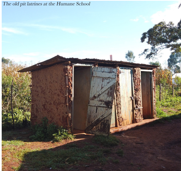
The old pit latrines at the Humane School
