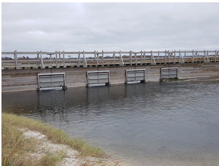
Figure 9: Sluice gates at Slusan. Photo by: Kristian Ångbäck
