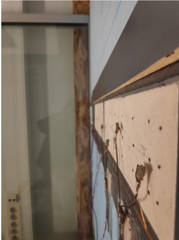
Figure 20 thermocouples on the heat-exchangers and outside near the fans
