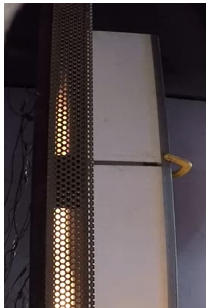
A11. f) Live Fire Test Perforated Cavity Obstruction under Fire
