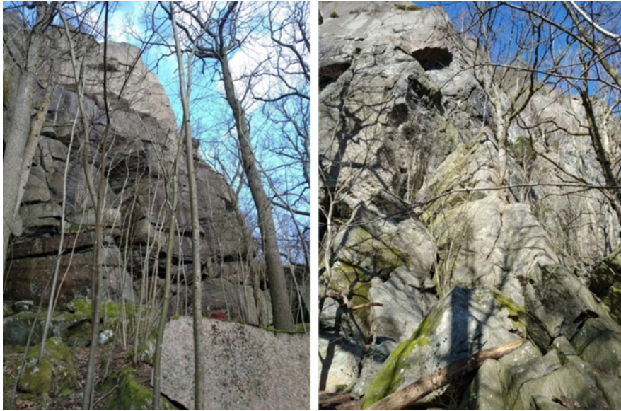
Fig. 24. Some of the climbing walls of Fjällbo. The discontinuities in the rock represent planes of weakness and thus potential rockfall sources.
