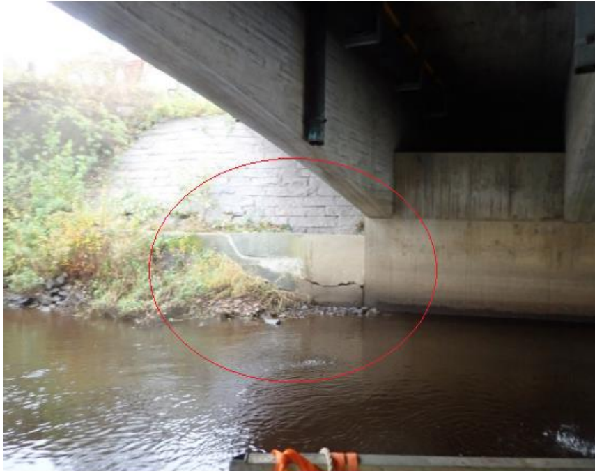
Figure 2.14.: Severe cracks in wing wall of the left abutment at Tegelbruksbron Bridge (MTE, 2020)
