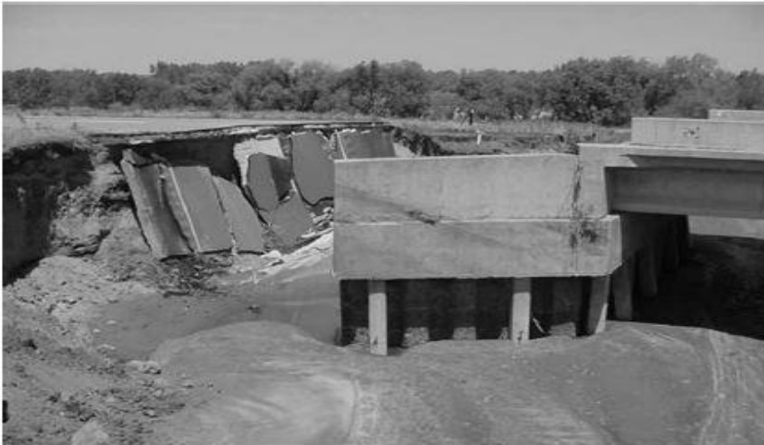
Figure 2.5.: Local scour formation at bed around an abutment of a waterway bridge (Ettema et al., 2004)
