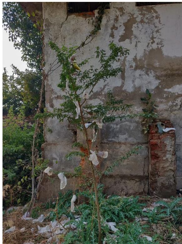
Figure 9 This picture shows the environment behind the girls' bathroom in the old building.
