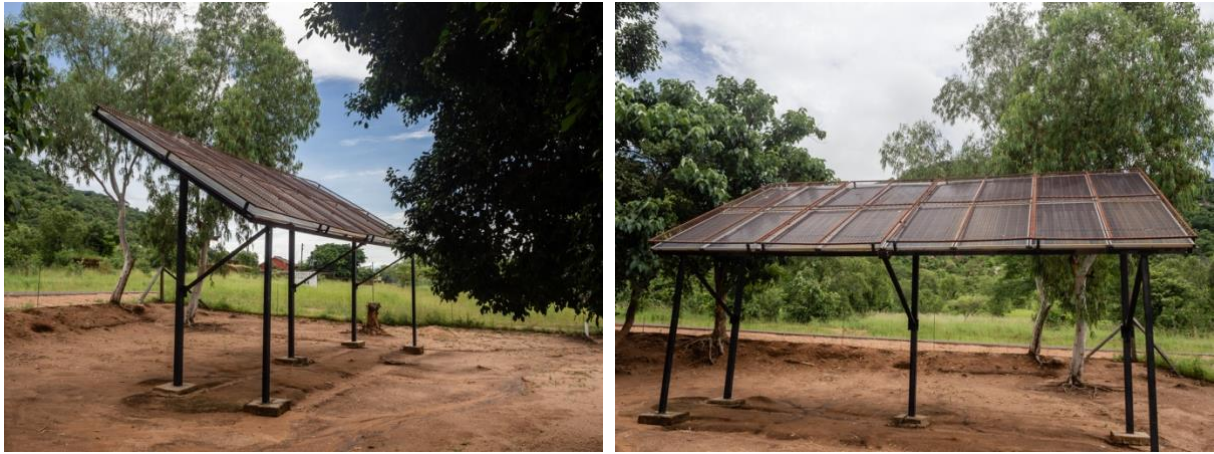
Picture 7 & 8: Solar micro-grid at clinic in Cape McClear from the side; Solar micro-grid at clinic in Cape McClear from the front. Cape McClear. Zoe Elsner.
