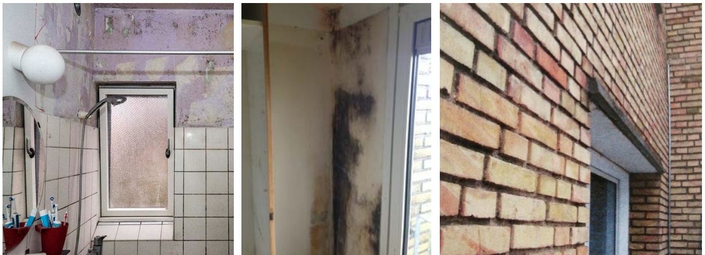
Figure 42: Tingbjerg: Example of severe mould formation in bathroom (left) and behind a built-in closet (middle); Example of eroded brick joints (right)
