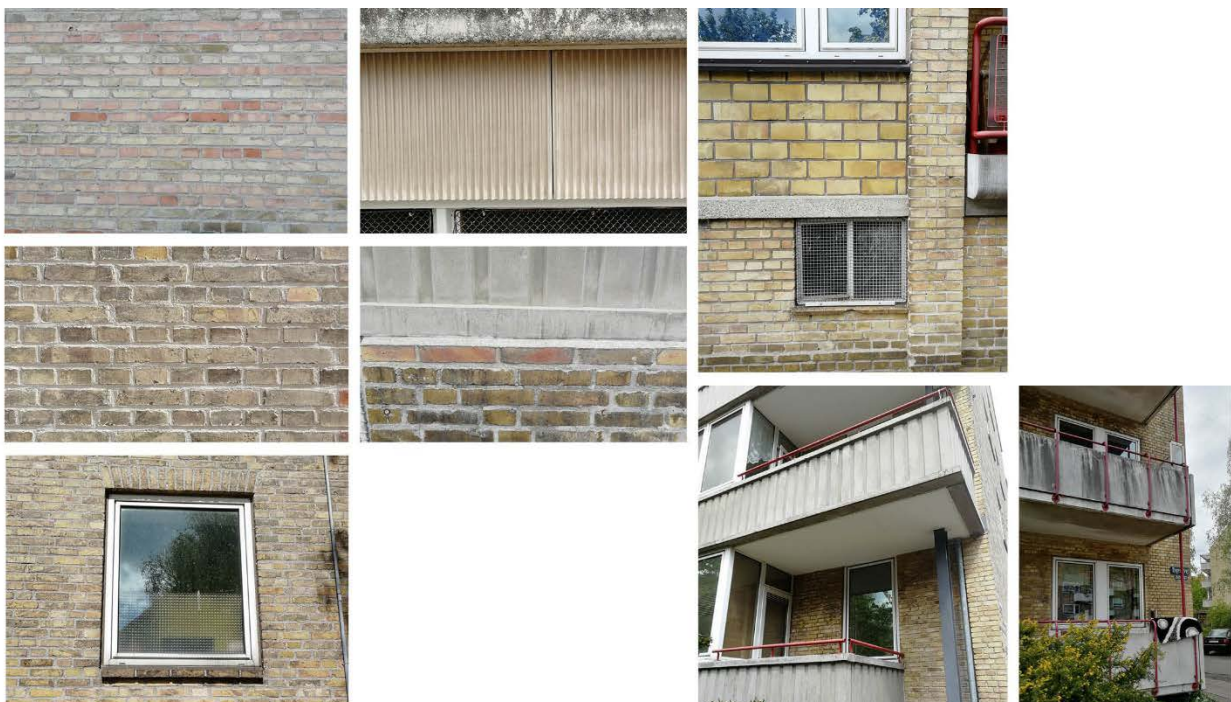
Figure 60: Existing materiality (1/2). Yellow brickwork, gray concrete elements and (mostly red painted) steel structures
