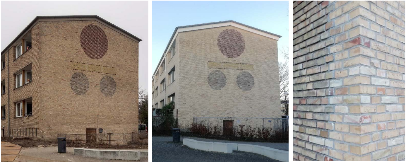
Figure 43: Tingbjerg: Original brick detailing at gable (left) and restored brick detailing after gables were insulated (middle); transition between original wall and re-built gable wall (right)
