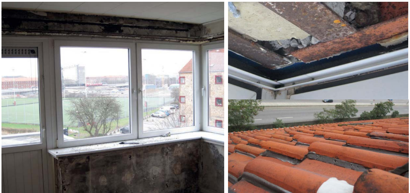
Figure 33: Lundevænget: Water and mould damages at a gable apartment (left), corroded steel beams (top right), reparations on original tiled roof (bottom right)
