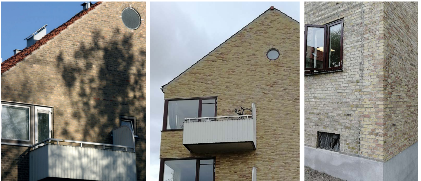
Figure 34: Lundevænget: Original gable wall (left), Insulated gable with new windows (middle), Transition between insulated gable wall and original wall (right)
