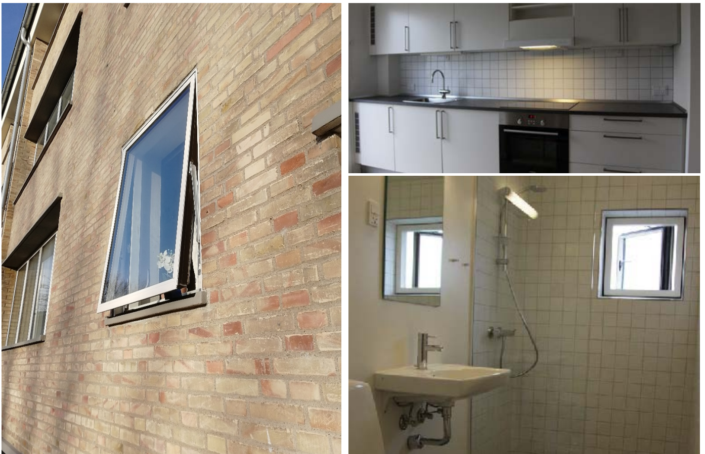
Figure 44: Tingbjerg: Repaired brick wall with repaired joints and new and slender window frames (left), Examples for new kitchens and bathrooms (right)
