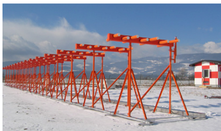
Figure 3.21: ILS antenna array consisting of multiple Log-Periodic Dipole Array (LPDA) antennas. [VHF Nav 2020]
