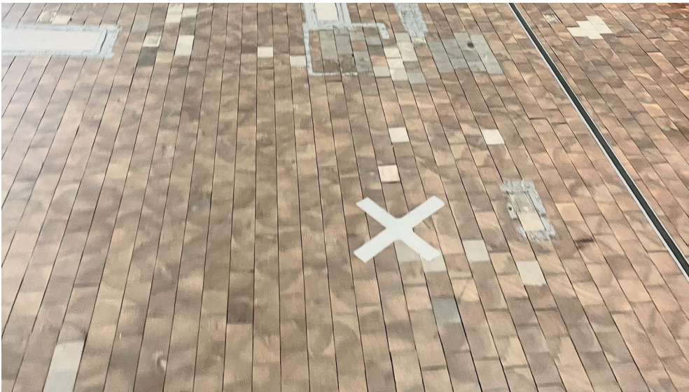
The floor inside Galleria Boulevard is mended by silver tape.
