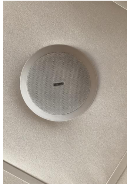
Figure 37 A recessed loudspeaker attached in a soft tile ceiling which is held up by radially extended arms above the ceiling. (Michael Lindberg)
