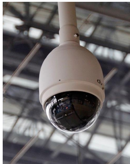
Figure 39 A surveillance camera mounted on a pole hanging down from the ceiling. (Peggy_Marco, 2015)
