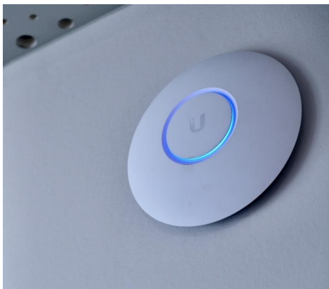
Figure 38 An access point for a wireless network is fitted using a bayonet mount onto a base plate. The ethernet cable is placed in a tailored cable hole on the backside of the access point. (Ihennen, 2020)
