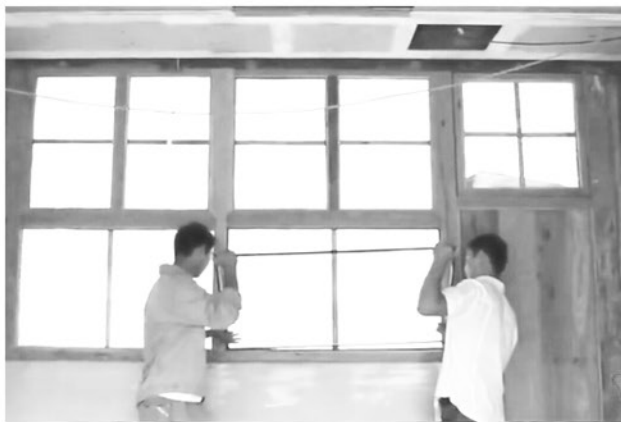
C PROBLEMS in restoring windows Bad thermal and sound insulation
