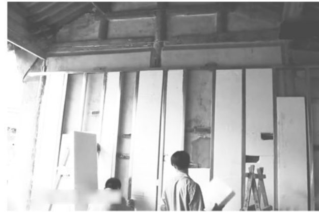
SOLUTIONS of the shared wall restoration The shared wall is thickened , and sound insulation cotton is added to obtain a better sound insulation effect.
