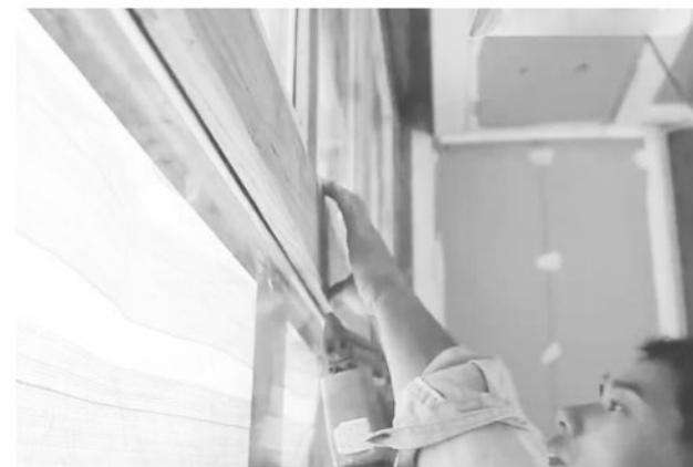
SOLUTIONS of windows restoration Under the premise of keeping the wooden windows frame , the original single-layer glass is replaced by the insulating glass to increase the sound and thermal insulation effect of the house.
